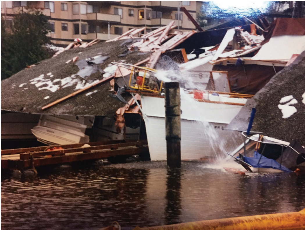
Meydenbauer Bay, 1998, when the weight of 15” of heavy snow crushed Dock B’s roof onto the boats. Shown is the Grandfar ’s bow prior to its extraction, and the beginning of a long and expensive process of renovation at the Vic Frank boatyard on Lake Union.
