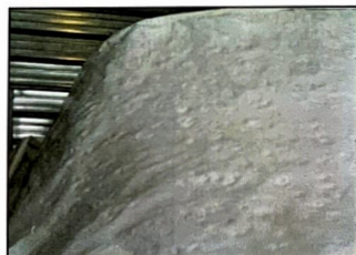
Hail damage- OUCH!! (photo by Skip Vashon)
